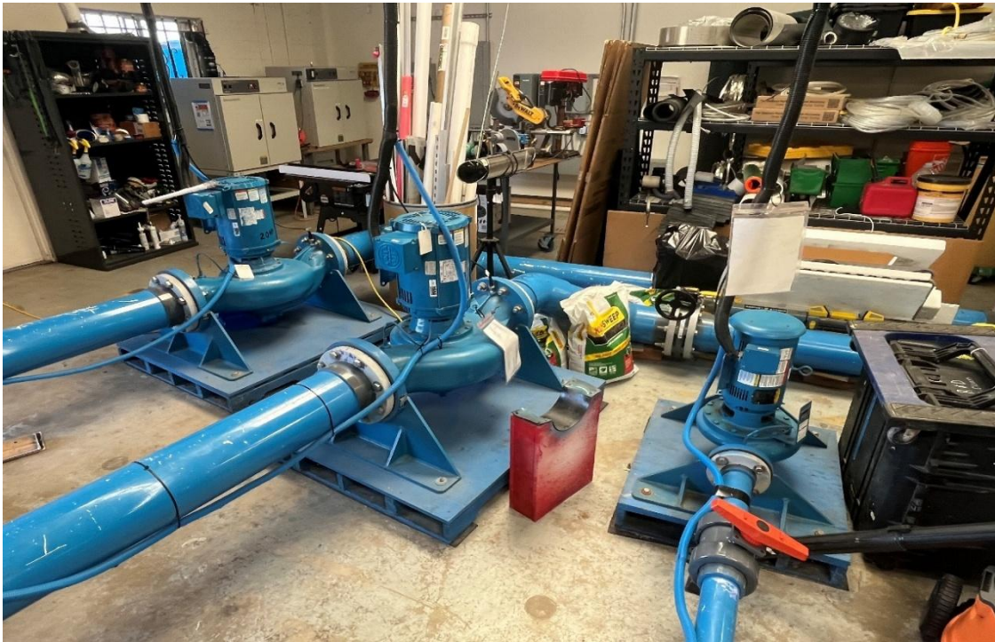
Figure 6: Test Loop Pumps
