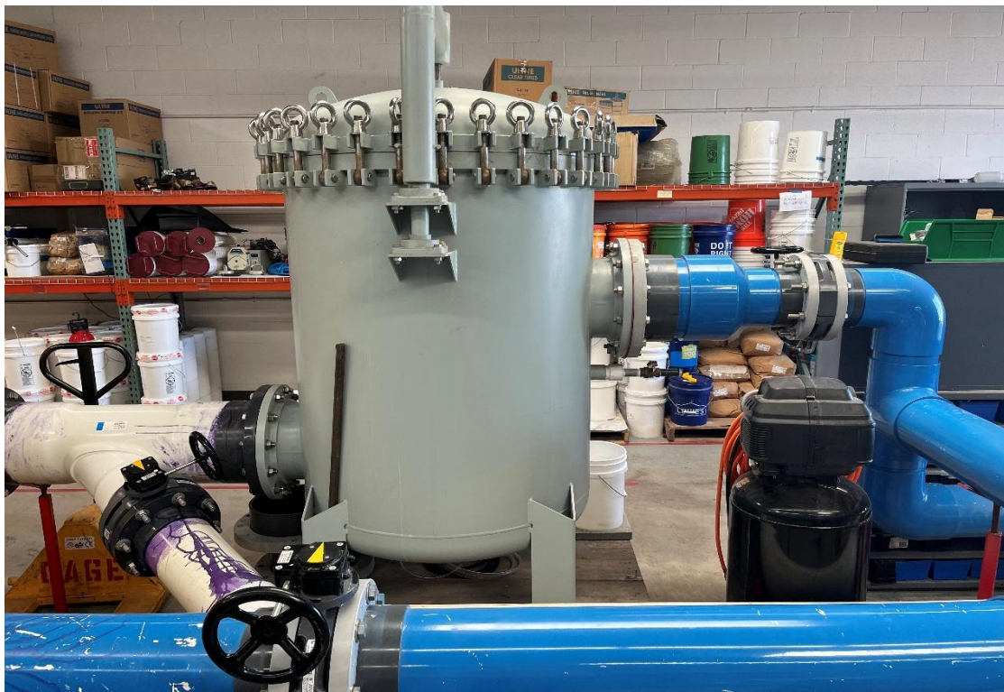
Figure 7: Test Loop Filter Vessel
