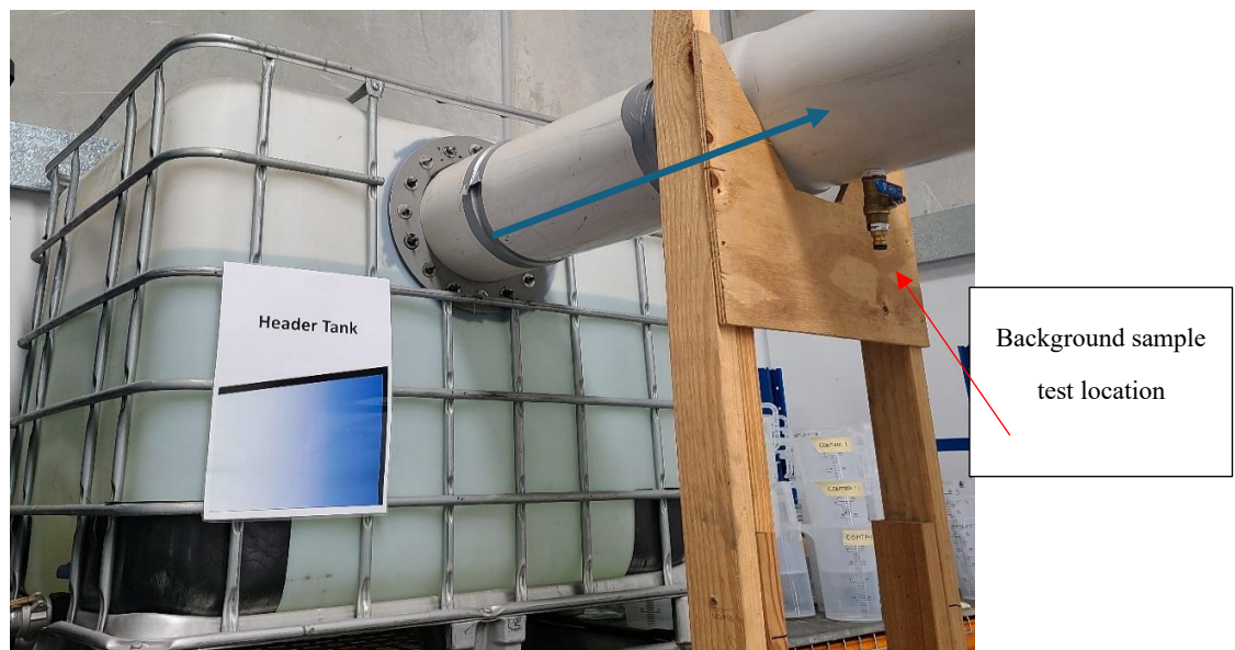
Figure 5. Photo of the Installed Constant Head Tank
