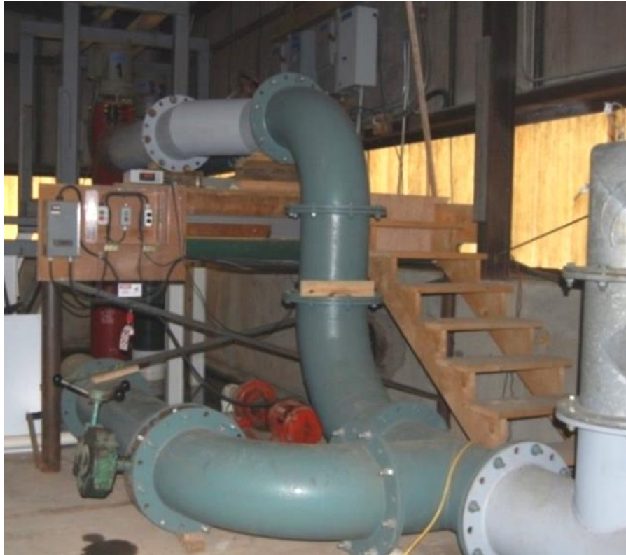
Figure 7 Photograph Showing Laboratory Pumps
