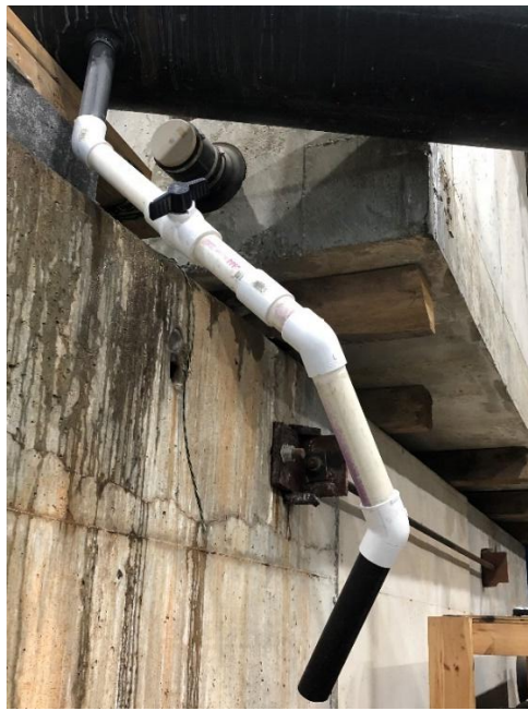
Figure 8 Photograph of Background Sampling Port
