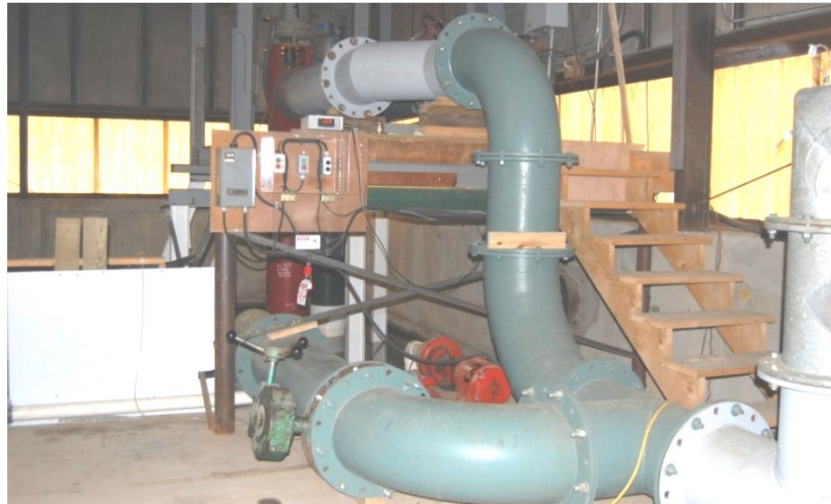
Figure 10 Photograph of Laboratory Pumps
