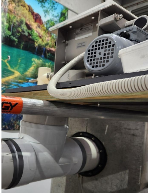
Figure 9 Upstream Dosing Location
