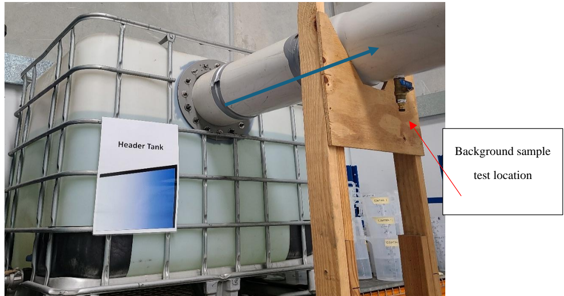
Figure 6 Photo of the Installed Constant Head Tank
