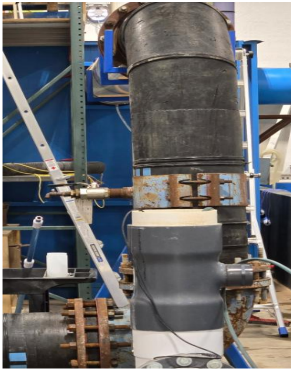
Figure 12 - Background Sampling Port Test Loop 2 and 3
