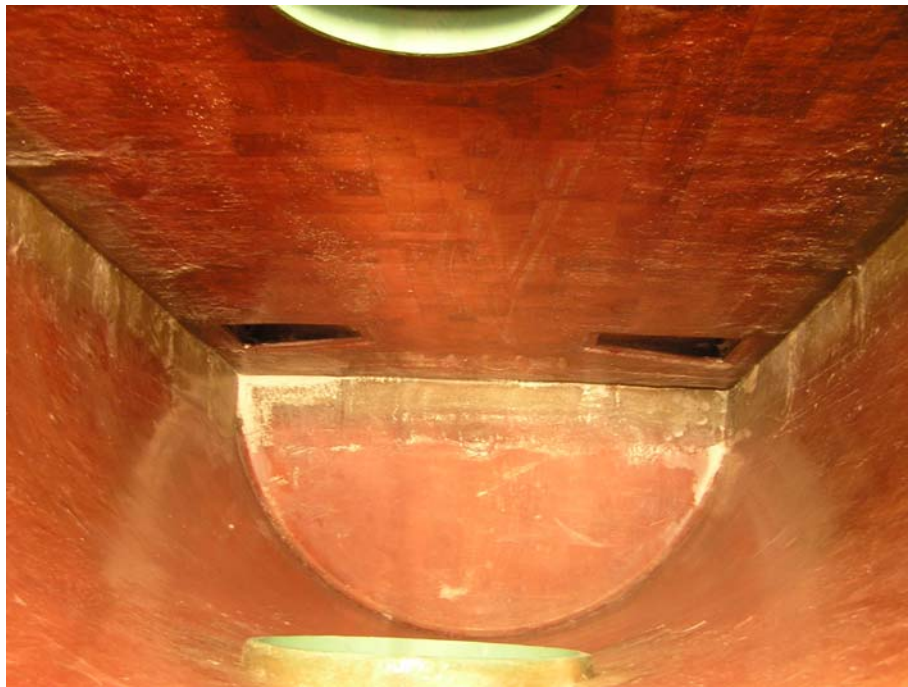
Figure 3 View of the baffle wall from the second compartment of the M2 manhole.
